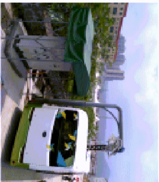
Figure 1. BYD Bus up overhead charging
