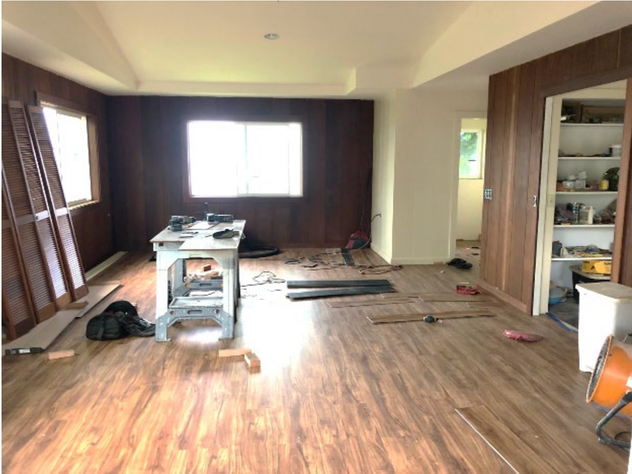
Figure 1. Newly renovated interior of the former Amy Greenwell house to become the “Hale o Pūlelehua” Community Center. Flooring, windows, fixtures, and ceiling have been replaced.
