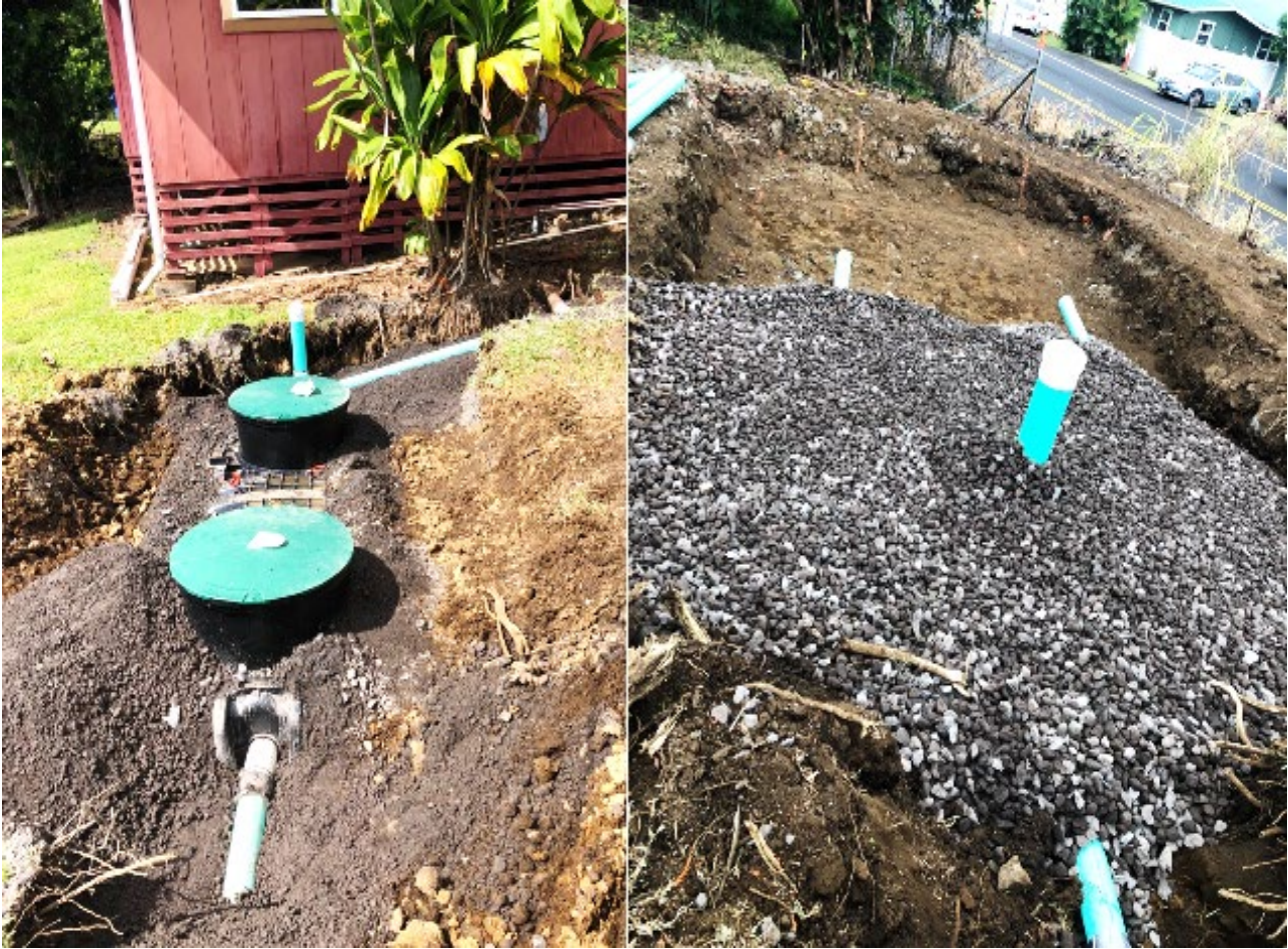
Figure 3.1 & 3.2. The original cesspool has been closed, and the new septic system has been installed and filled for public safety.
