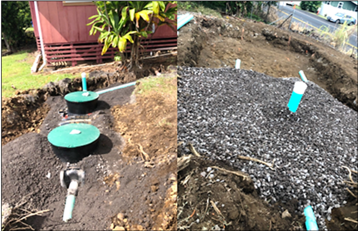
Figure 3.1. The original cesspool has been closed, and the new septic system has been installed and filled for public safety.
