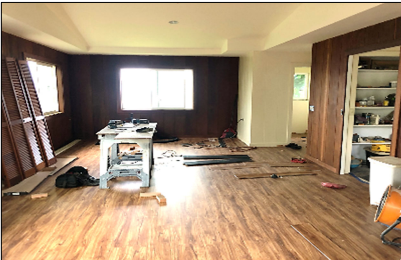
Figure 1. Newly renovated interior of the former Amy Greenwell house to become the “Hale o Pulelehua” Community Center. Flooring, windows, fixtures, and ceiling have been replaced.
