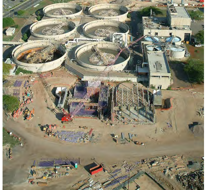
The Sand Island 82-mgd Wastewater Treatment Plant (WWTP) is the State of Hawaii's largest, serving metropolitan Honolulu. Beginning in 2006, RMTC provided the design for two upgrade and modernization projects totaling over $70 million in construction cost.
