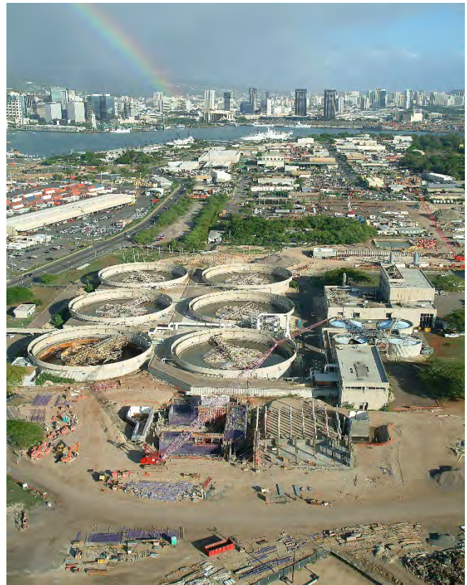
RTMC was program manager for the City and County of Honolulu's $350-million-dollar upgrade of the Sand Island WWTP and related facilities within the Sand Island Basin.
