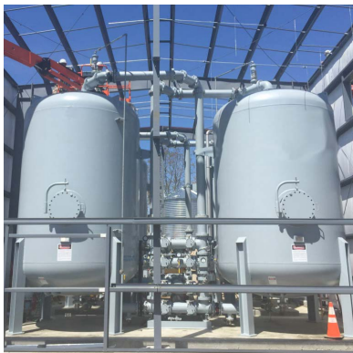
We vetted and tested technologies and oversaw design of a system that is now providing clean drinking water.
