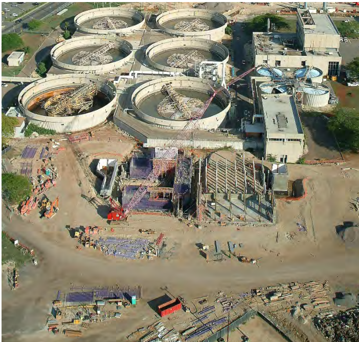
The Sand Island 82-mgd Wastewater Treatment Plant (WWTP) is the State of Hawaii's largest, serving metropolitan Honolulu. Beginning in 2006, RMTC provided the design for two upgrade and modernization projects totaling over $70 million in construction cost.
