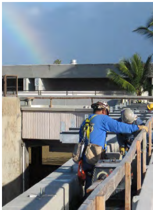
Air Conditioning Modifications, Phase II, Diamond Head Chiller Plant and Common Chilled Water Loop, HNL, Oahu (2009)
