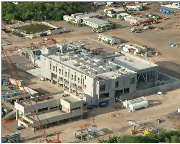
Sand Island Wastewater Treatment Plant Ultraviolet Disinfection Facility and Pump Station, Oahu (2006) Construction Cost: $81M
