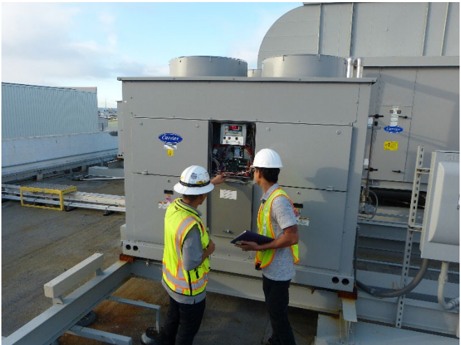
Air handlers for HVAC system inspection
