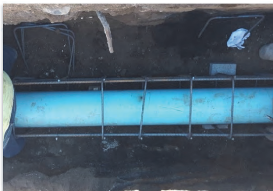
Installation of new 8-inch sewer line within the intersection of Punchbowl Street and Queen Street
