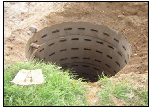
Visual inspections of well and casing are conducted monthly to check for any or other potential problems
