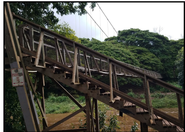
When water levels are too high, residents park along Menehune Road and cross using a pedestrian bridge
