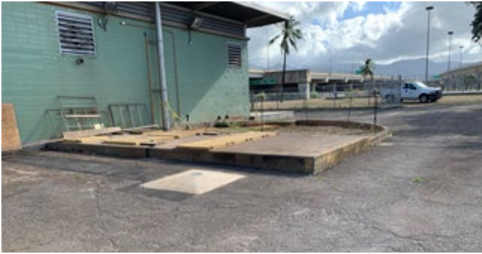
Pump Station and Wet Wells
