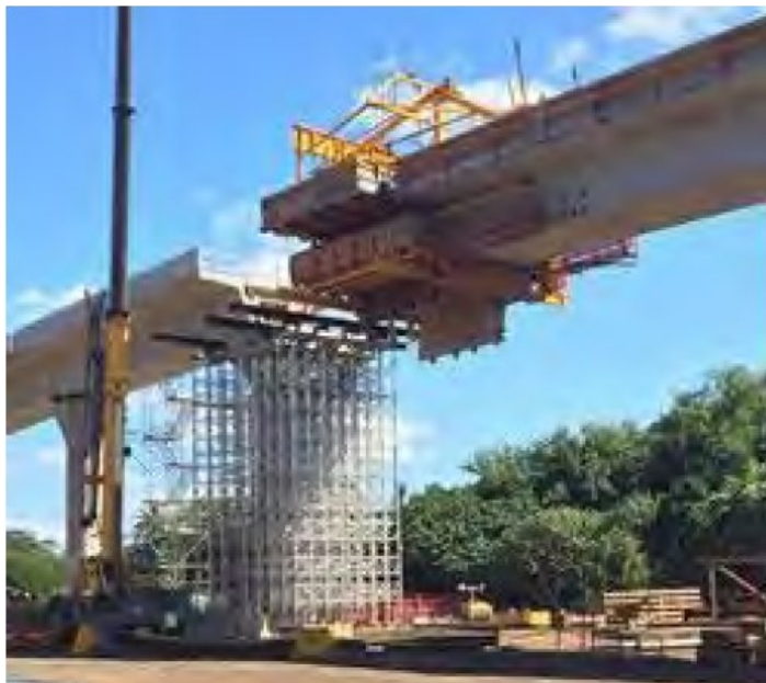
Typical rail guideway section under construction from East Kapolei. Jacobs managing the environmental compliance and coordinating activities under the historic preservation program.
