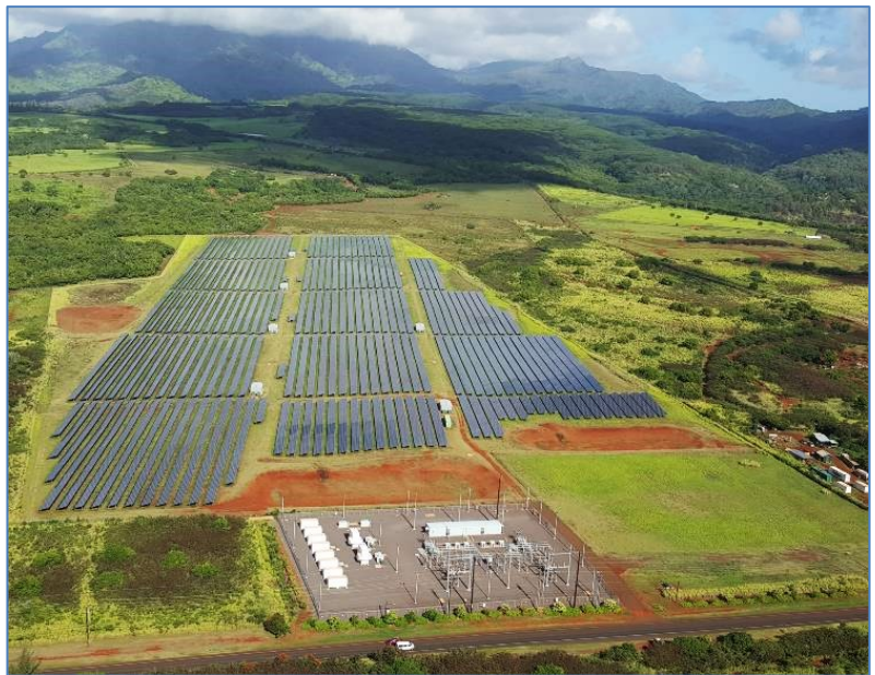
Completed Anahola Solar Project.
