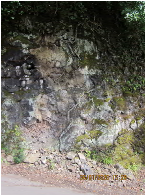
Photo 6. Transect F-W-04, Central Section. Note the rockfall on upslope side of road.
