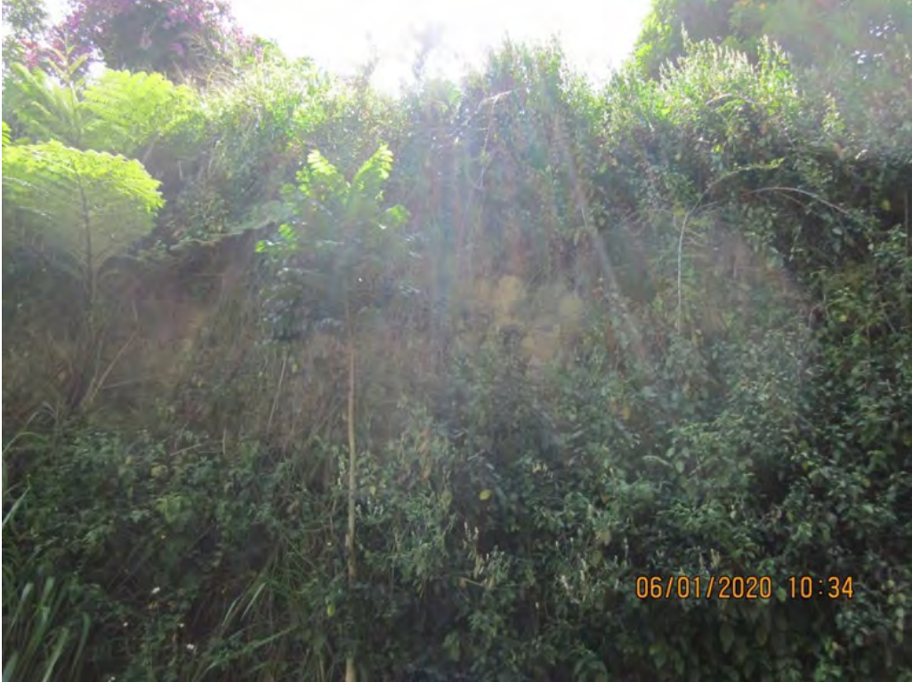
Photograph 3. Partially-vegetated road cut slope with exposed soil in upper slope area.
