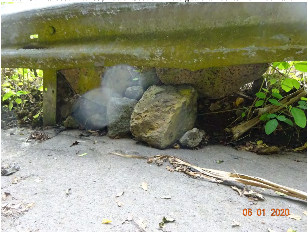
Photo 14. Transect F-W-05, Lower Section. Note previous rockfall makai side of road.
