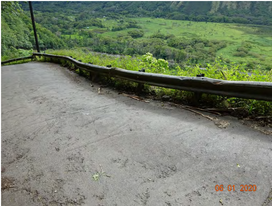
Photo 13. Transect F-W-05, Lower Section. Note guardrail dents from rockfall.
