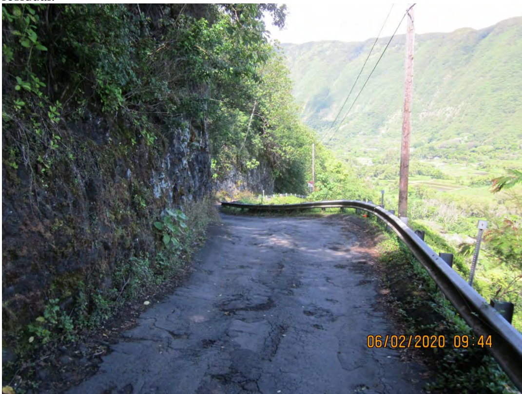
Photo 16. Transect F-W-06, Lower Section. Note the steep upslope and road deformation.
