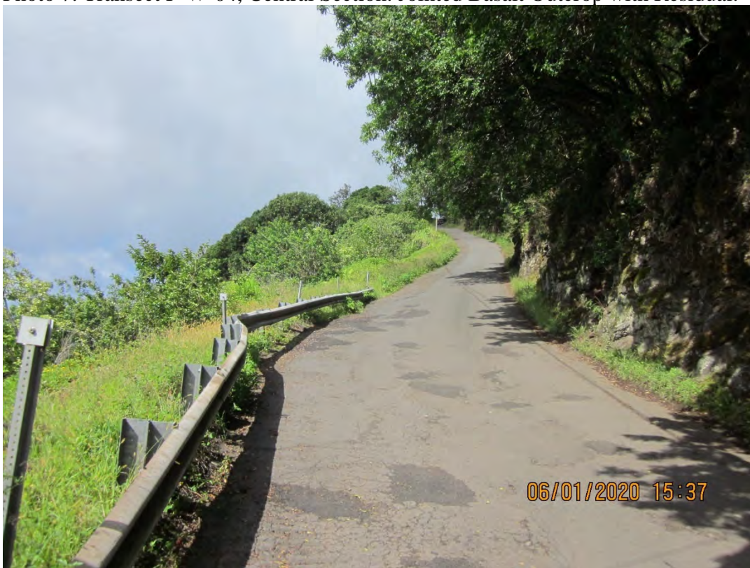
Photo 8. Transect F-W-04, Central Section. Guardrail strike from boulder or vehicle.
