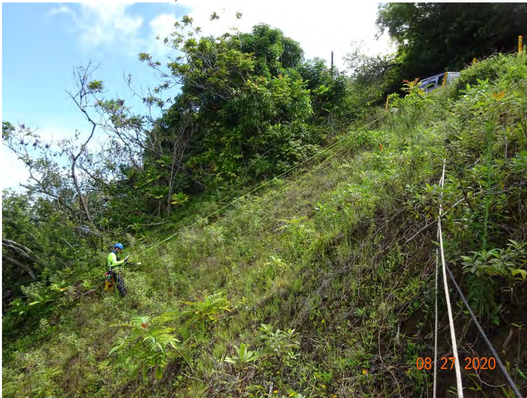
Photo 26. Transect F-W-04, Central Section. Rappel work at slide area.
