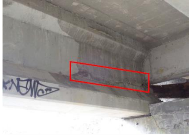
Delaminated area measuring approximately 4' long x 10" high occurring in downstream fascia of Girder 1 at North abutment.
