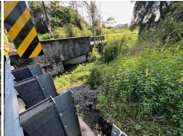
Photo 2: Problematic area needing additional clearing post-storm events.
