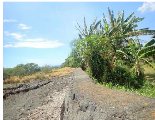
Vegetation encroachment on private property along the Pa'auau Channel.
