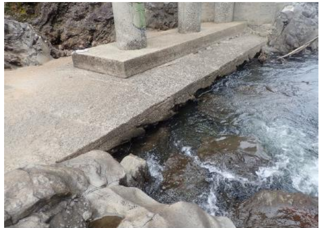
Erosion and undermining of the south fascia of center pier scour protection.
