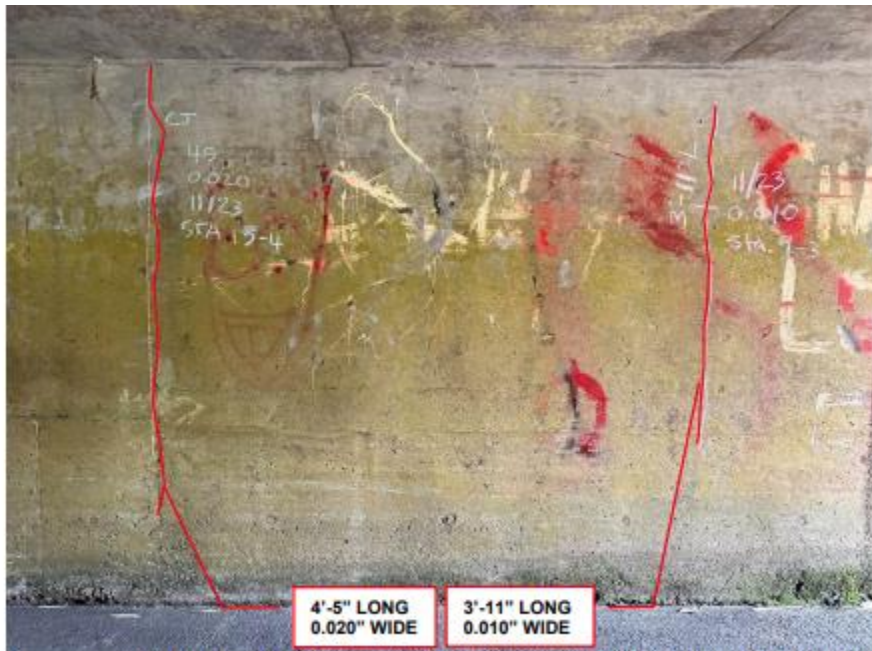
PHOTO 18 CELL 1 WALL 1 @ 9'-3" AND 15'-4" FR UPSTRM END: 0.010" AND 0.020" WIDE, 3'-11" AND 4'-5" LONG (CS2) VERTICAL CRACKS, 2 FT = CS2 1130
