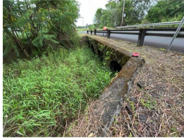
Bridge #24-5 Ainalako Road Culvert: Excessive vegetation on NBI road culvert.
