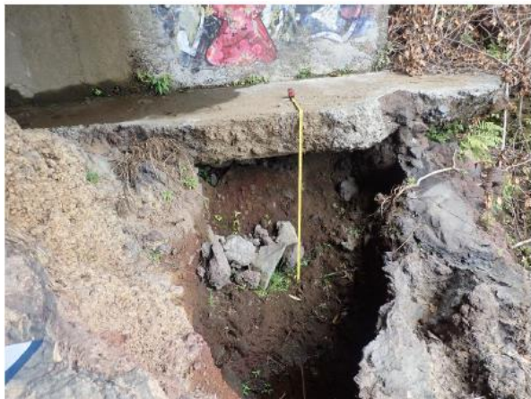
The downstream end of North abutment footing/scour protection exhibits undermining measuring approximately 10' long x 4' high x 5'-6" deep.
