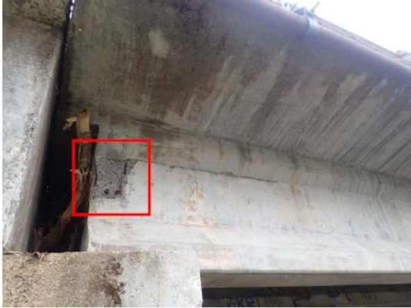
Concrete spall measuring approximately 12" long x 14" high x 1.5" deep, with exposed reinforcement (minor section loss observed).
