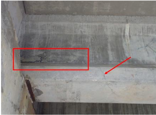
Delaminated area measuring approximately 30" long x 10" high occurring in the upstream fascia of Girder 2 at North abutment with diagonal crack measuring up to 0.04" wide occurring in web and bottom flange of girder.
