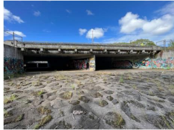
Bridge #24-6 Komohana Street Bridge - Waiakea Stream Bridge: Graffiti may impact inspections.
