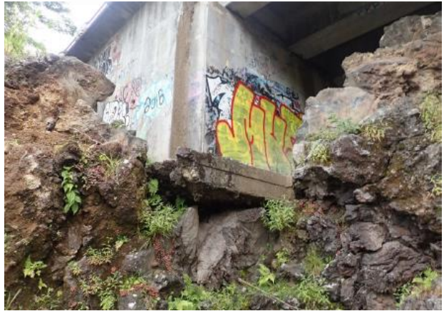
Upstream end of North abutment footing/scour protection exhibits undermining measuring approximately 6' long x 5' high x 4'-6" deep.
