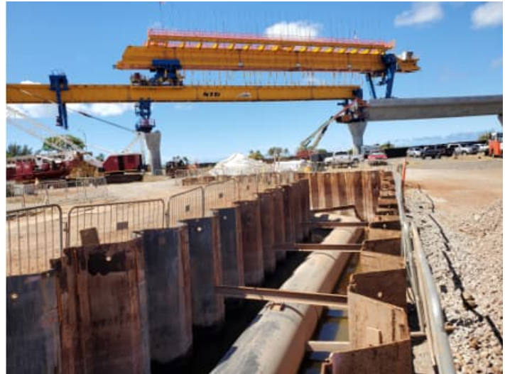
Jacobs maintained operation of the WWPS while constructing a major pipeline through reclaimed land and coordinated with ongoing construction along the alignment.
