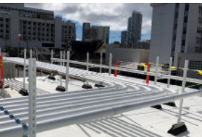
1411 South King Street New Electrical Services
