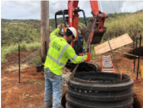
HECO Kahe-Halawa/Kahe-Waiiau 138 kV Replacement
