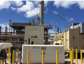
Hawaii Gas SNG Facility Above Ground Storage Tank
