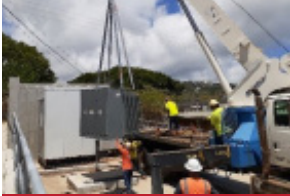
HBWS Emergency Generators at Kalihi, Halawa and Kunia
