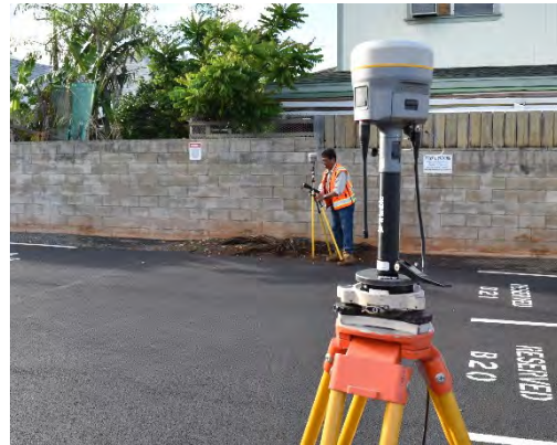
RMTC surveyors conduct field surveys utilizing the latest in GPS technology: the Trimble R10 GNSS System.
