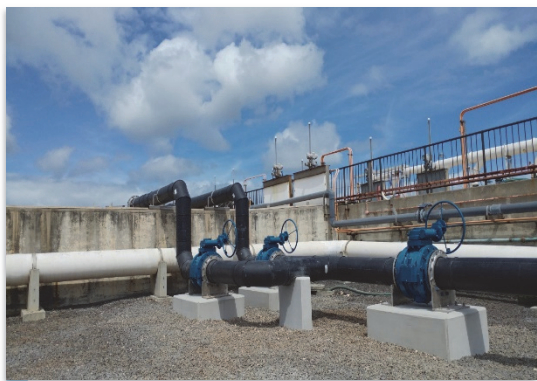
12-inch HDPE force main discharge valve manifold terminating into the Pre-Aeration Channel
