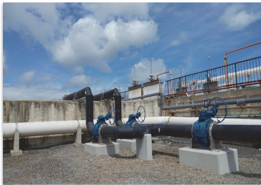
12-inch HDPE force main discharge valve manifold terminating into the Pre-Aeration Channel
