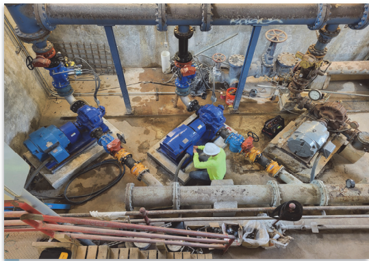
New irrigation pumps at Kahuku Agricultural Park
