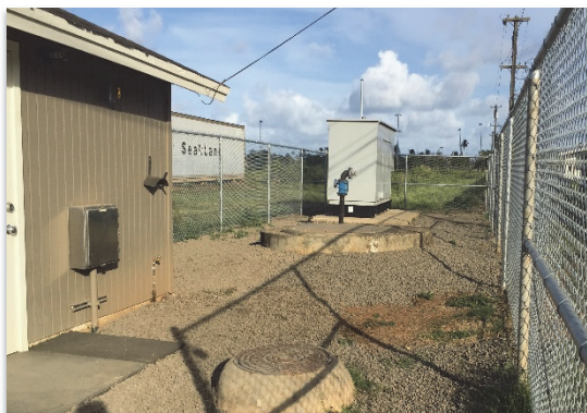
Upgraded pump station building and new diesel generator
