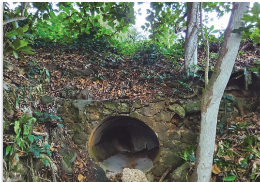
Drainage culvert in need of repair along Old Kalaniana'ole Road
