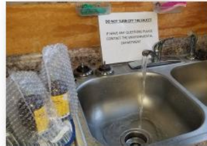
Faucet purge prior to sampling
