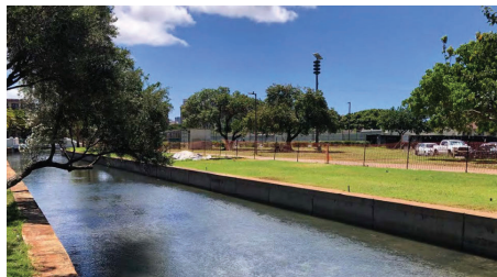
Ala Moana Regional Park Improvements. The collapsed wall on far side of the existing canal was replaced with mechanically stabilized earth wall with geosynthetic reinforcement.
