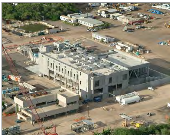
Sand Island Wastewater Treatment Plant Ultraviolet Disinfection Facility and Pump Station, Oahu (2006) Construction Cost: $81M
