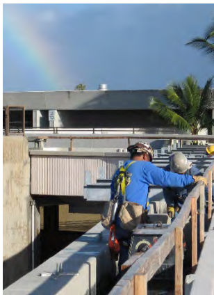
Air Conditioning Modifications, Phase II, Diamond Head Chiller Plant and Common Chilled Water Loop, HNL, Oahu (2009)
