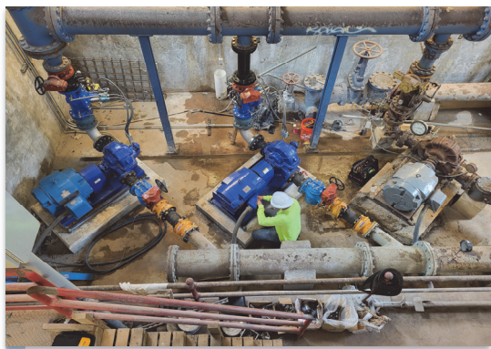
New irrigation pumps at Kahuku Agricultural Park
