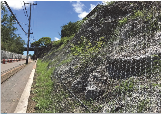
Wire mesh slope stabilization system
