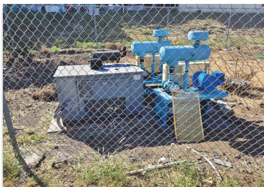
Existing aerobic treatment unit at 'Ouli 'Ekahi
