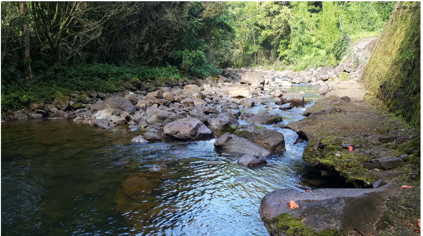
B8: Scour/undermined on the inlet side at the upstream end.
