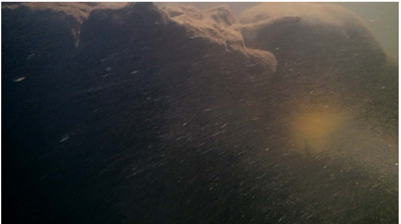
B16: SOUTH ABUTMENT (UNDERWATER) Underwater photo below the rock at the upstream side (Refer to photo B7).
