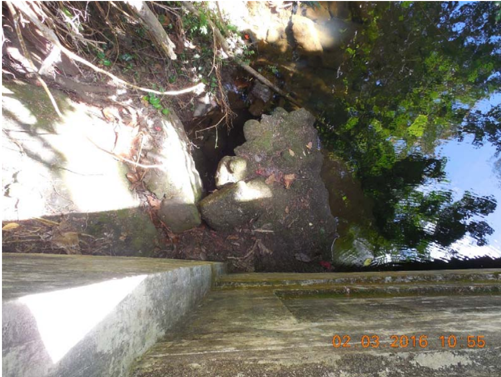
B13: Scour/undermined condition on the outlet side downstream end at the north abutment.
