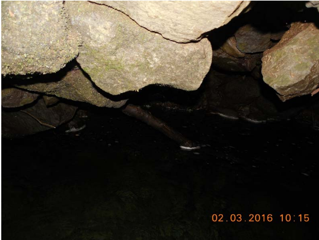
B11: Close up of the scour/undermined condition inlet side at north abutment upstream.
