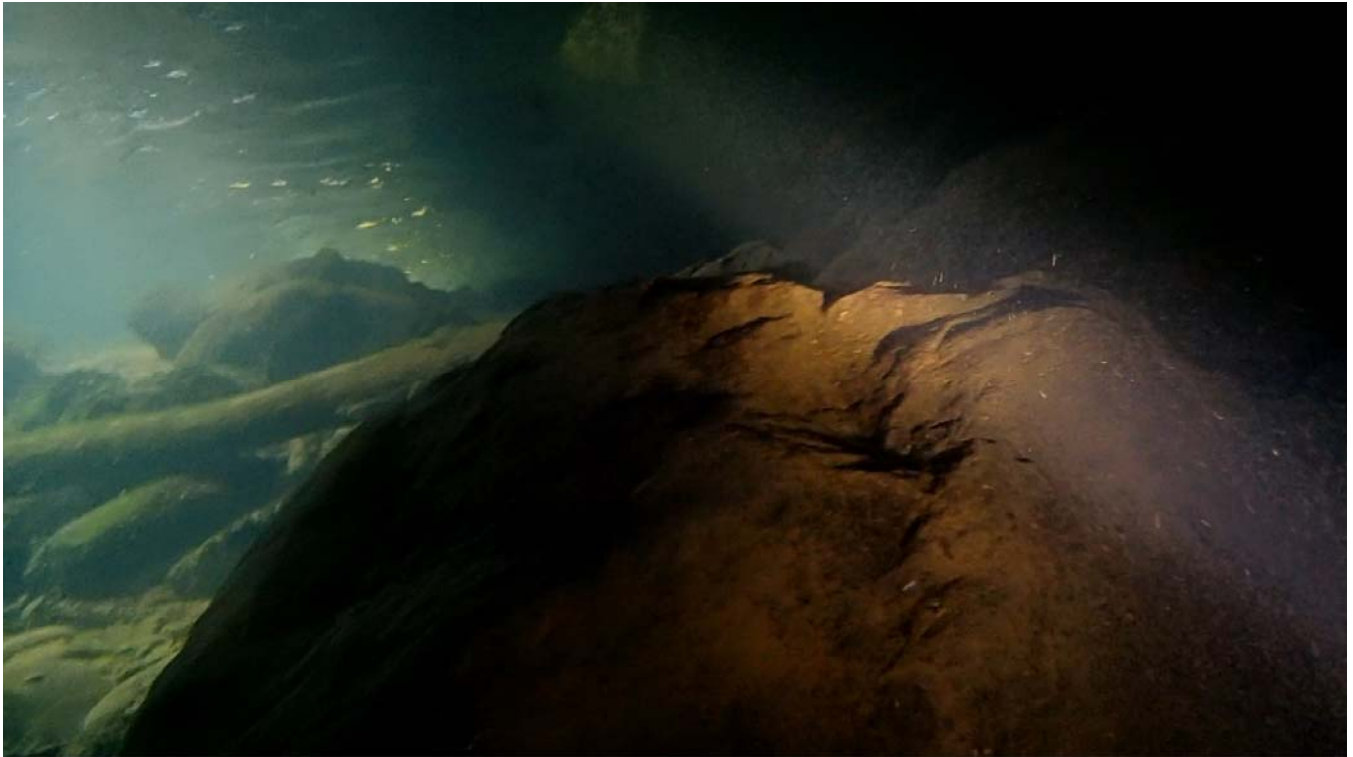
B19: NORTH ABUTMENT (UNDERWATER) Near the center of undermining upstream-side of north abutment.
