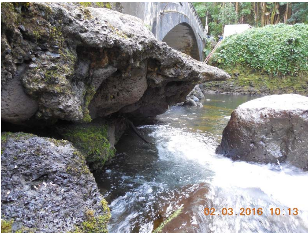
B10: Scour/undermined condition below the rock ledge inlet side at north end of bridge.
