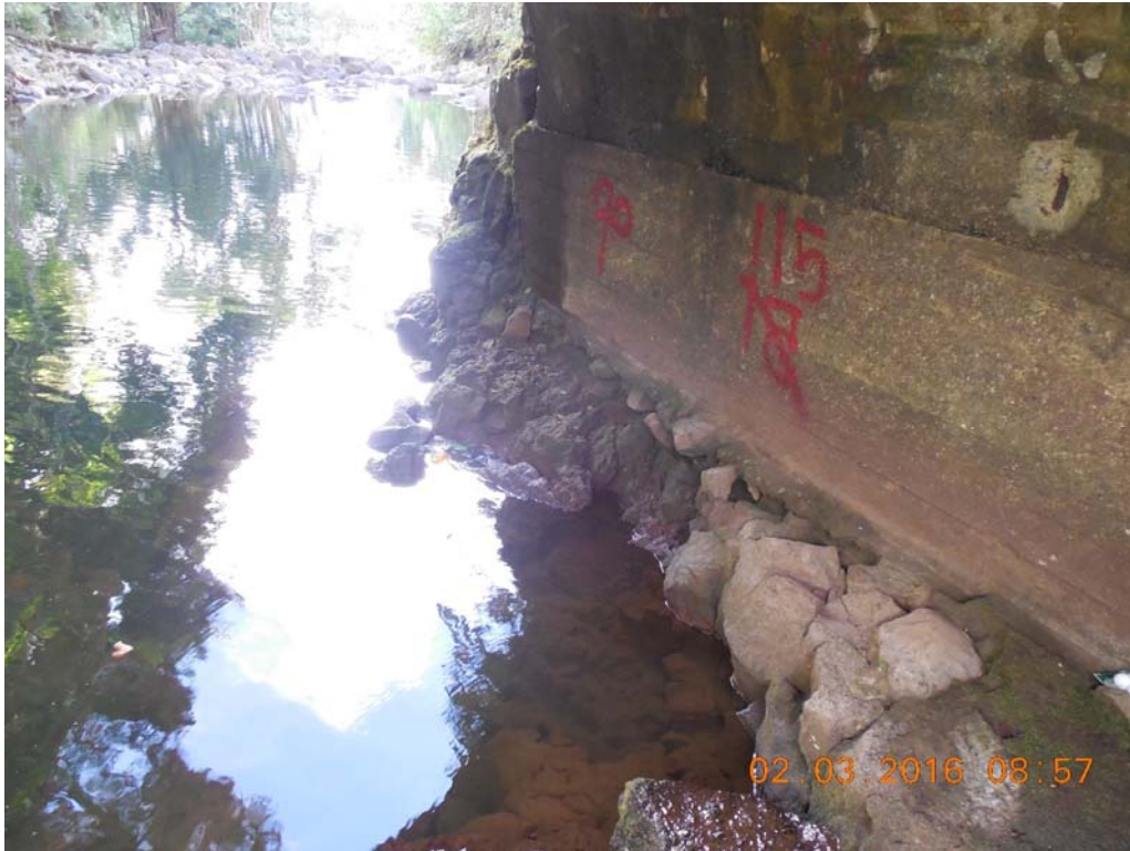
B15: Signs of minor scouring/erosion at the downstream side on the south rock ledge.
