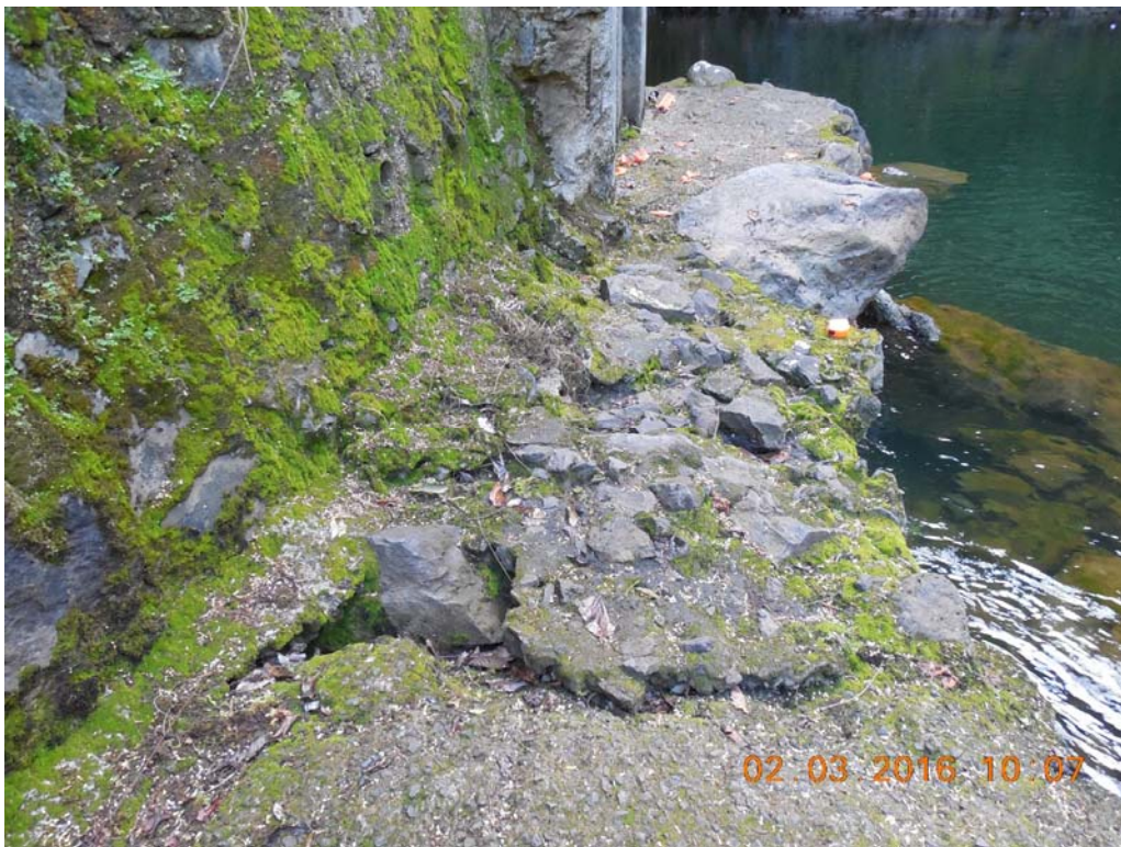
B14: Fractured cracks and erosion on upstream rock ledge north end. See North Abutment Plan on page 28 for location.
