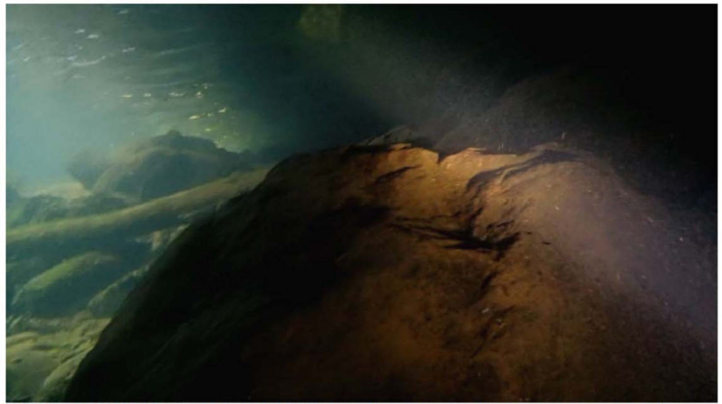
319: NORTH ABUTMENT (UNDERWATER) Near the center of undermining upstream-side of north abutment.
