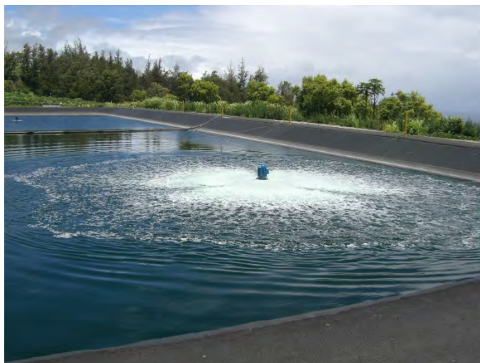
Figure 4-4. High Speed Floating Aerator
