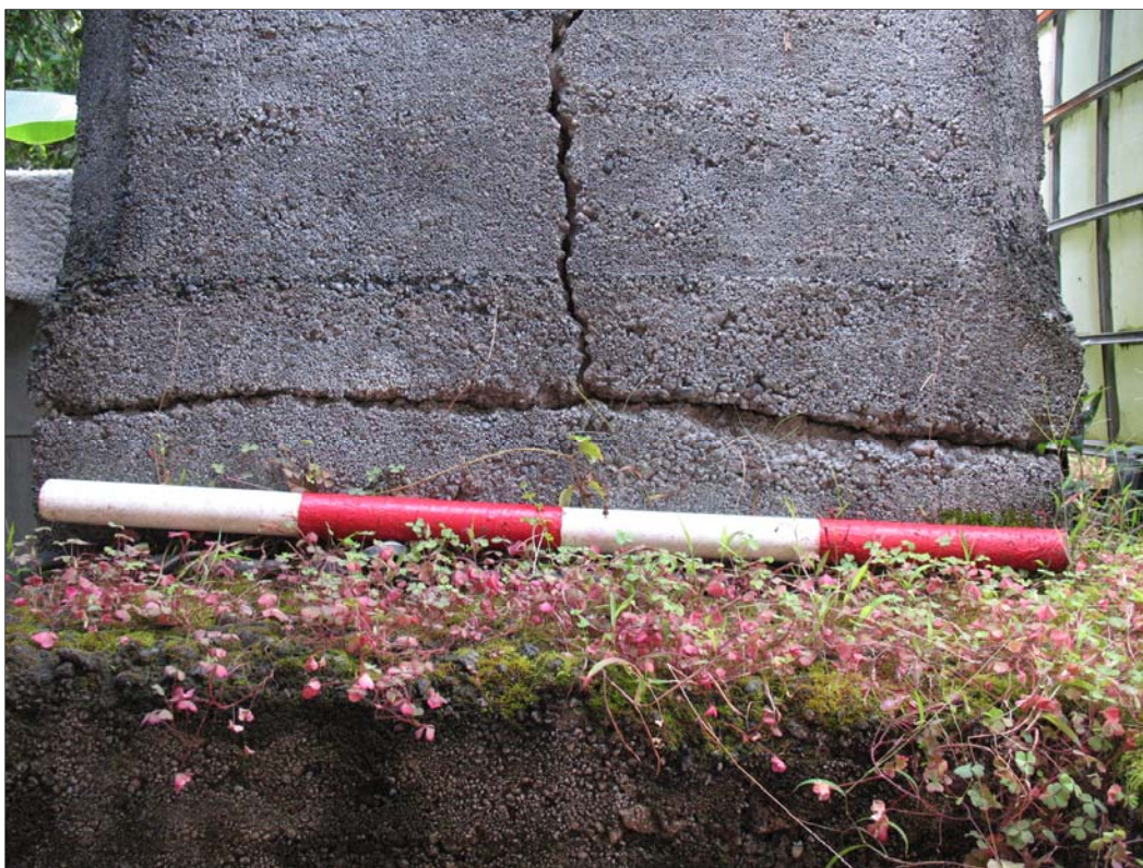
Figure 174. SIHP Site 30134, showing fractures near base of smokestack.
