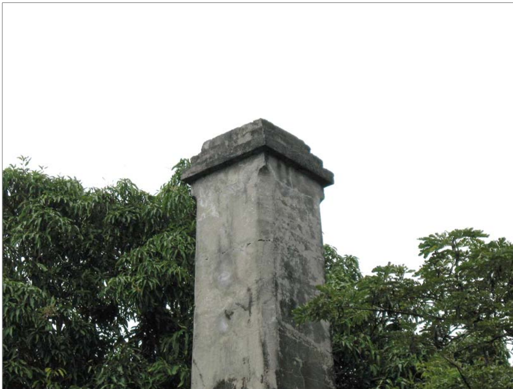
Figure 64. SIHP Site 2511 smokestack tower showing chamfer detail and missing cap.
