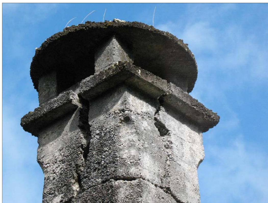
Figure 173. SIHP Sites 30134, circular smokestack cap, note the numerous cracks and fractures.
