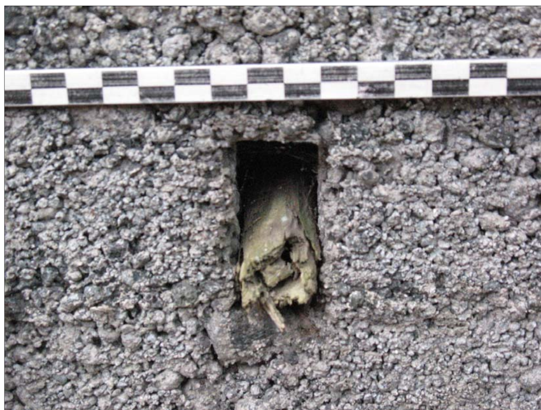
Figure 68. SIHP Site 2511 fragment of wooden tie still present in wall.
