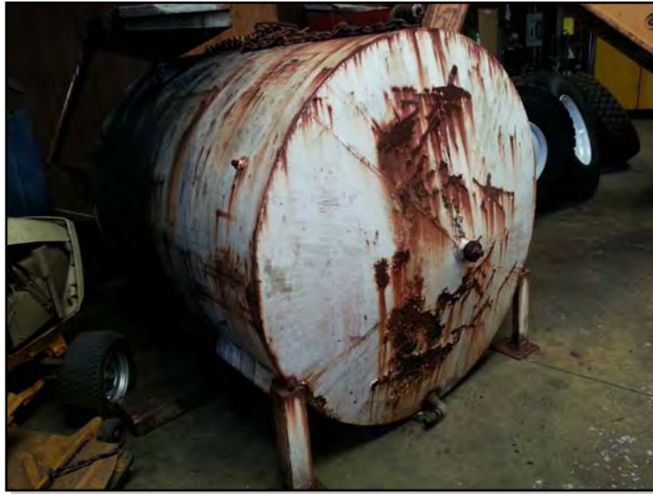
Photograph 9. A view of the AST within the warehouse of the subject property (October 30, 2012).
