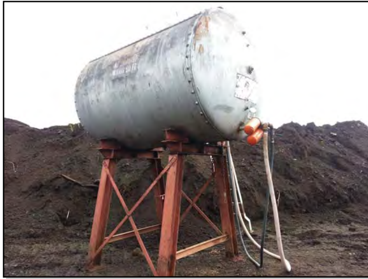
Photograph 49. A view of an old diesel AST on the adjoining property to the north of the west end of the subject property, TMK 1-5-007:007 (October 30, 2012).
