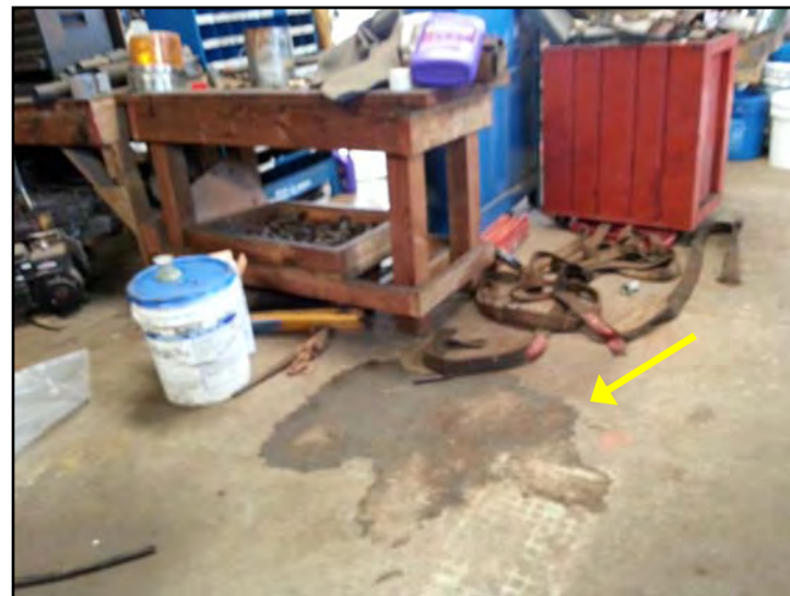
Photograph 8. A view of staining on the concrete floor within the warehouse of the subject property (October 30, 2012).
