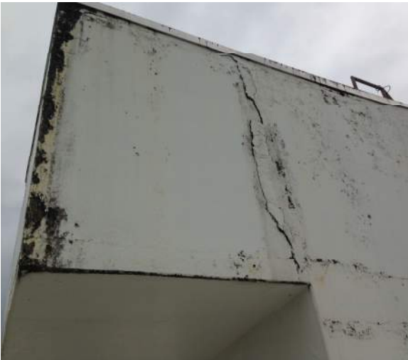
Photo 7: IMG_2491 – Spalling and cracking at Elevator Room
