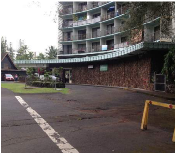
Photo 3: IMG_2447– Deteriorated pavement at drop off area
