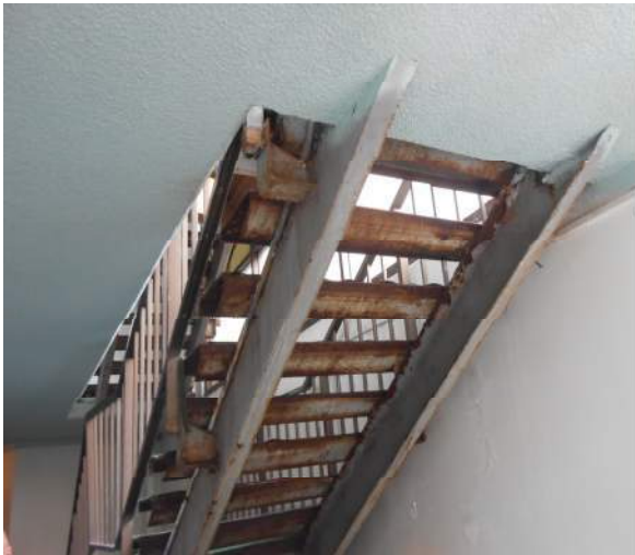
Photo 11: DSCN0481– Typical steel stair rusting
