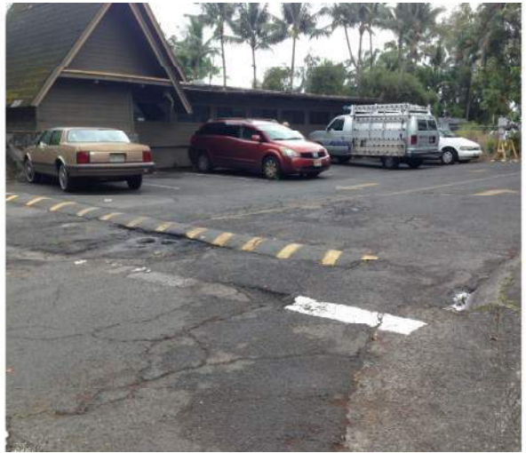
Photo 2: IMG_2445 – Deteriorated pavement at entry parcel
