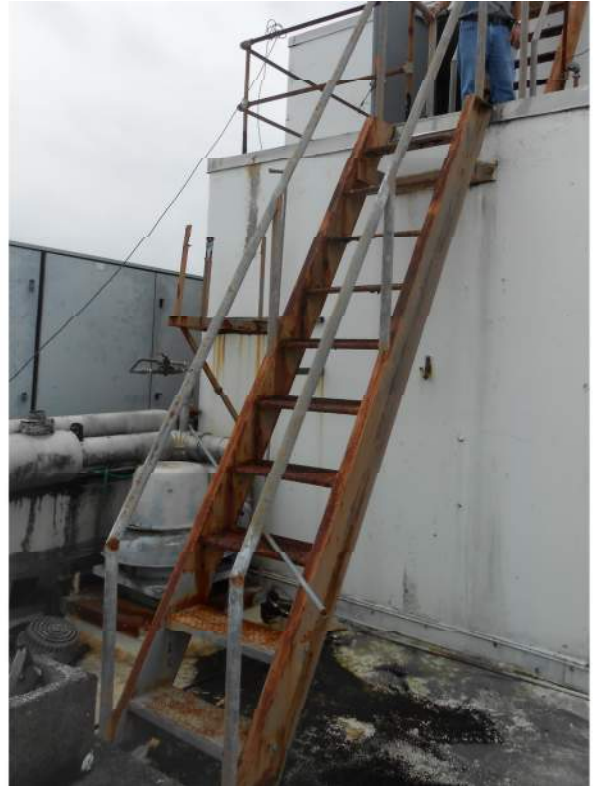
Photo 10: DSCN0471 – Roof stair rusting
