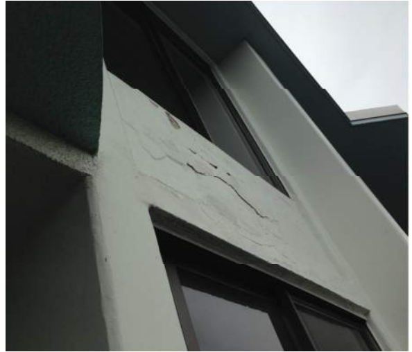
Photo 6: IMG_2523– Spalling at Exterior Wall
