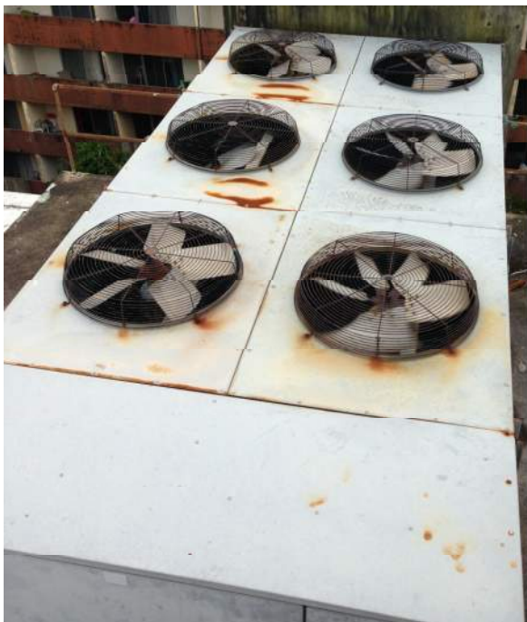
Photo 15: IMG_2489 – Air cooled chiller unit
