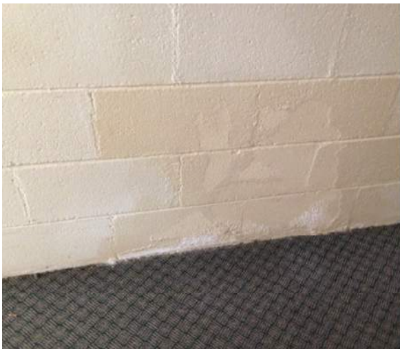
Photo 7: IMG_2297 - Efflorescence and Cracking/Patching in Hallways
