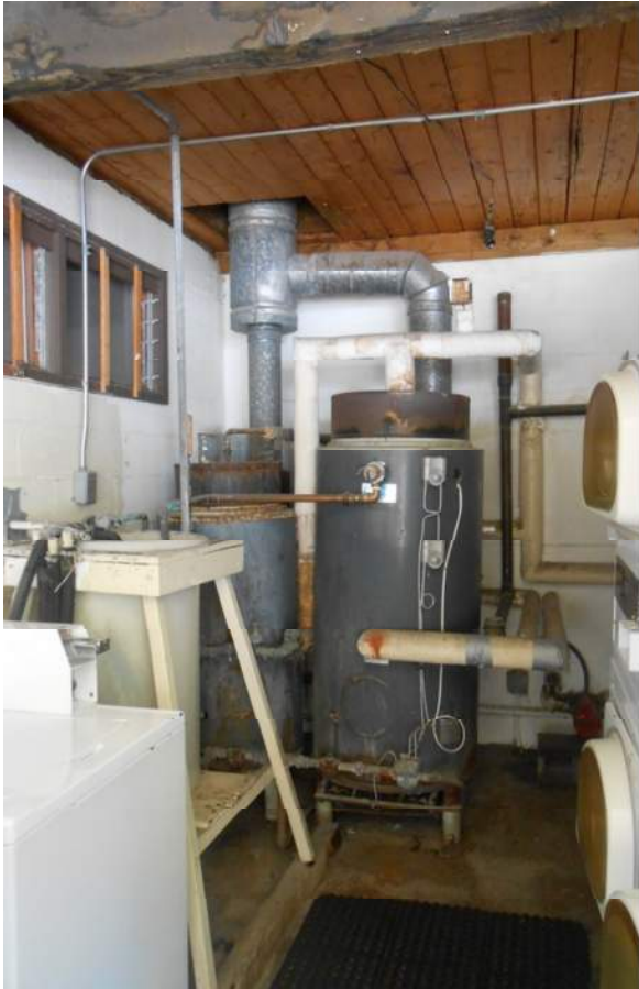
Photo 21: DSCN0423 – Hot Water Heater
