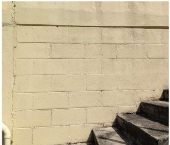
Photo 8: IMG_2283 – Cracking at Exterior Basement Wall.
