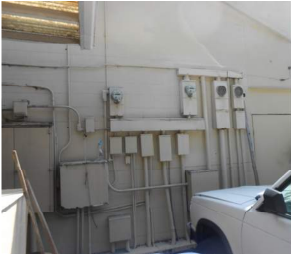
Photo 19: DSCN0424 – Electric Meters
