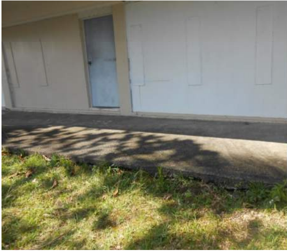
Photo 1: DSCN0429 – Undermining at Makai South Building Sidewalk
