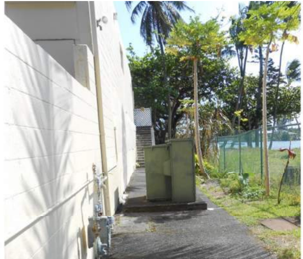
Photo 20: DSCN0426 – HELCO Transformer
