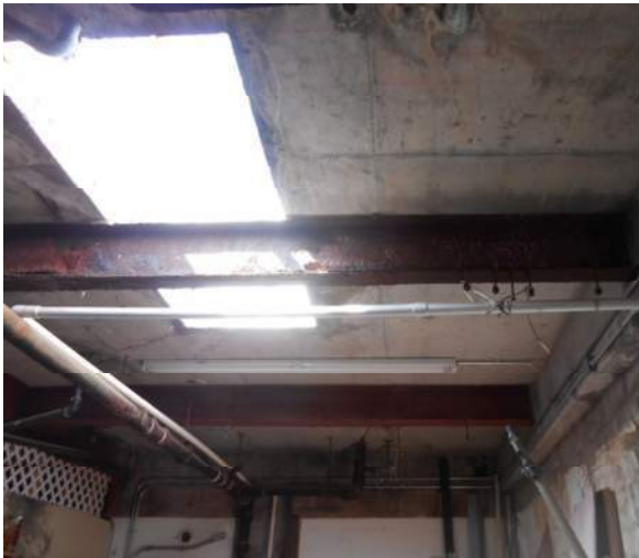
Photo 11: DSCN0415 – Section Loss at Steel Beam due to Corrosion
