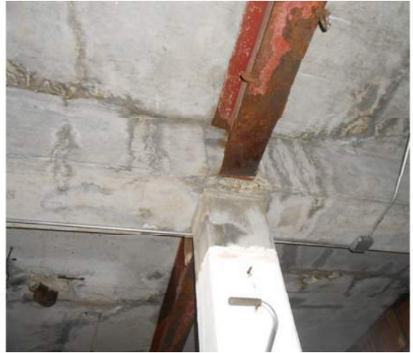
Photo 10: DSCN0420 – Spalling in Concrete Beam
