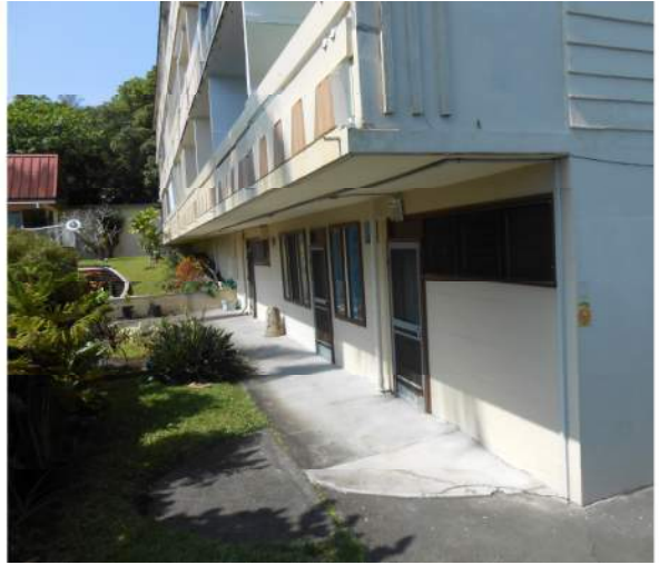
Photo 2: DSCN0438 – Cracking in Walkway
