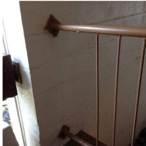
Photo 16: IMG_2296 - Railing Missing Bolt and Vertical
