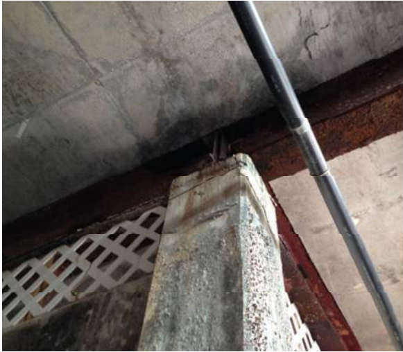
Photo 9: IMG_2269 – Cracking at Top of Column
