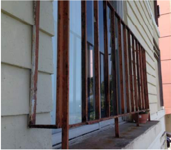
Photo 17: IMG_2300 – Rusting Railings at East End
