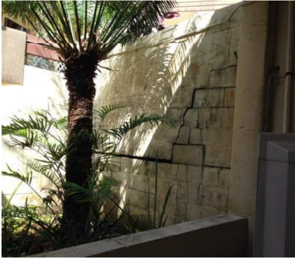
Photo 5: IMG_2278 – CMU Wall Failure
