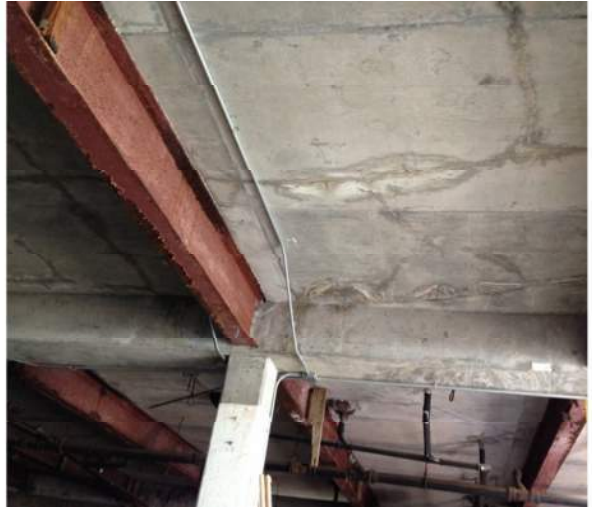
Photo 6: IMG_2276 – Cracking, Staining and Efflorescence at Restaurant Basement
