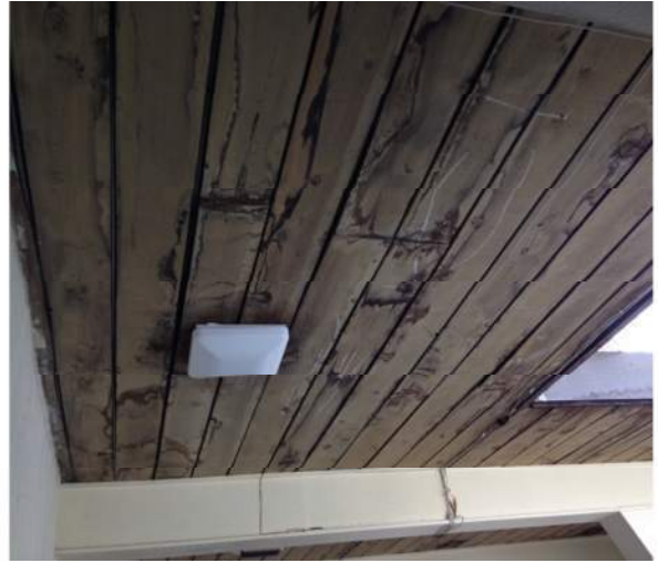
Photo 14: IMG_2306 Water Staining at Underside of Lobby Area Roof
