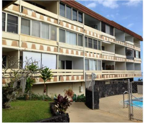
Photo 18: IMG_2264 – Typical Railing Condition
