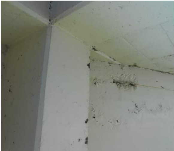
Photo 15: DSCN0428 – Spalling at Exterior Stair Soffit
