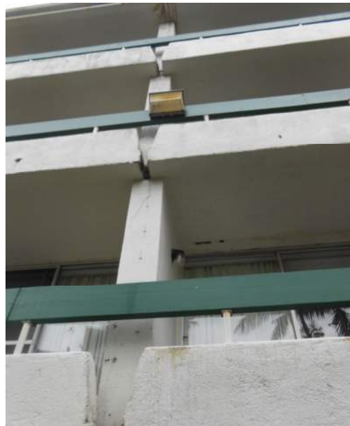
Photo 8: DSCN0501 – Cracking at Exterior Balcony Wall
