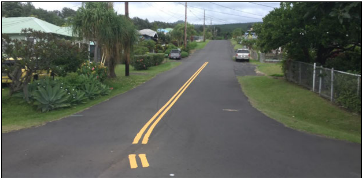
Figure 27. Photo looking up Ilima Street; note drainage in grassy shoulder on right side of photo; view to northwest
