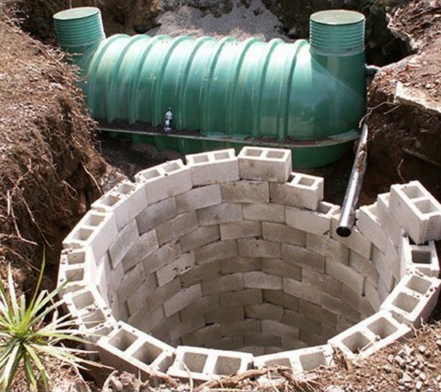
Orengo 1,500-gallon tank and block-lined seepage pit
